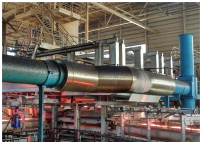
Existing end-fired regenerative furnace
